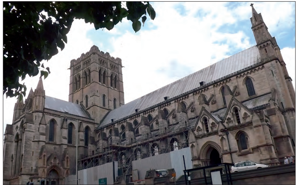
Work has started to replace the lead roof on the north side of the Cathedral following the receipt of a £180,000 grant from the World War One Memorial Trust
