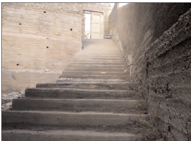
Entrance doors are difficult to open
